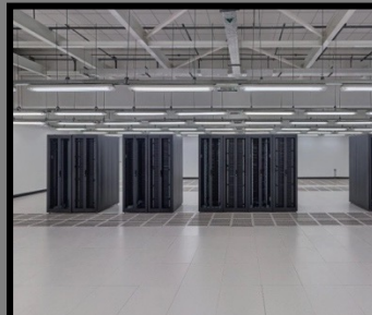
Data Centre - Abu Dhabi
